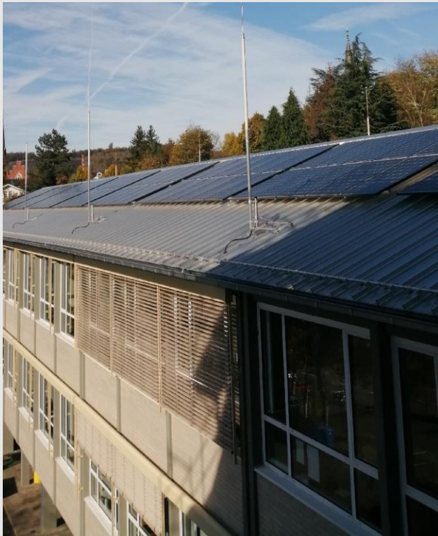
Solar panel on the roof top.
